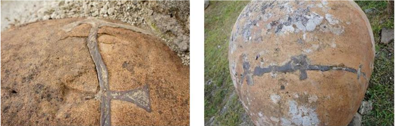
Fig. 6: Sub-Project 4: Dolium repair. Left: lead crack filling and tenons on large dolium . Right: iron crack filling and filling of cut for cross piece of staple (?) on small dolium .
